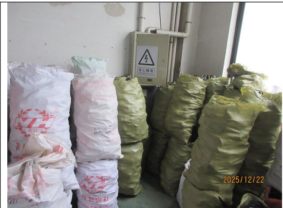
7-13 Electricity box was blocked by the flammable material
