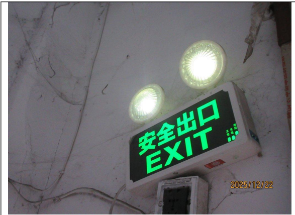
Emergency light testing
