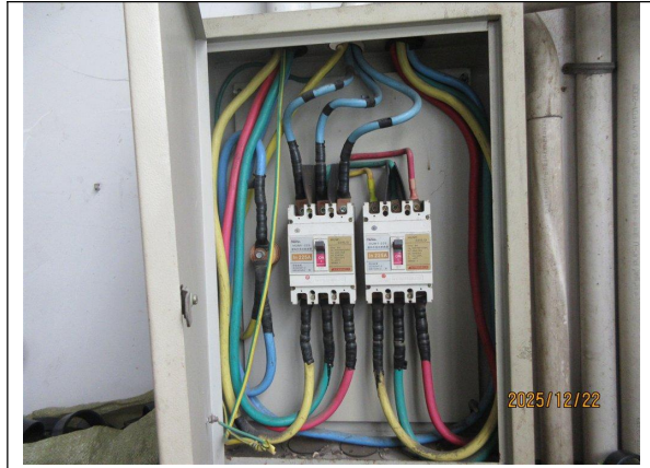
7-13 Electricity box were kept open, and without inner cover
