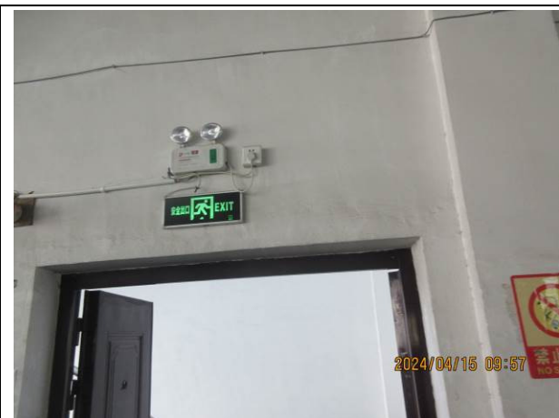
Exit sign and emergency light
