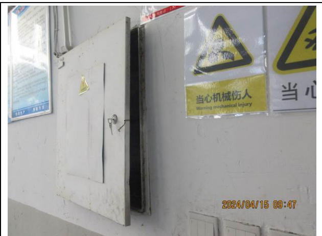
NC7.13 The outer protection covers of 20% distribution boxes were not locked
