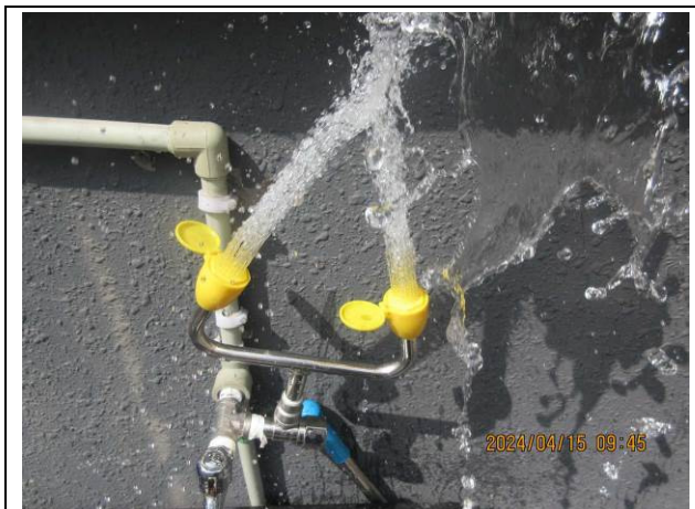
Eye washing facility
