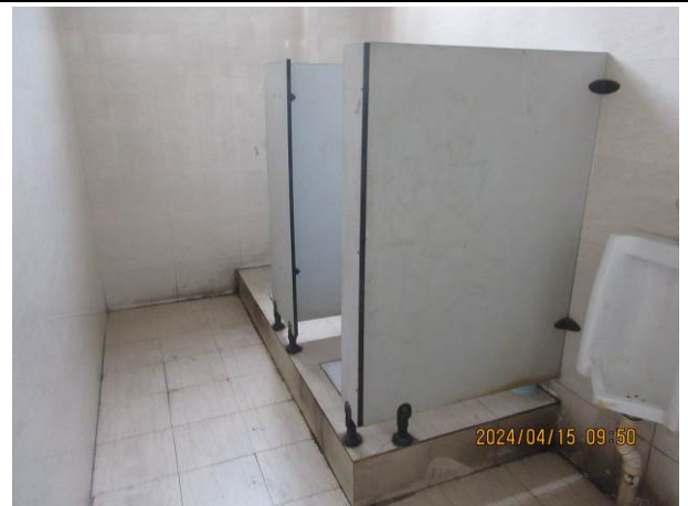
NC7.22 Toilets at workshop missed private door
