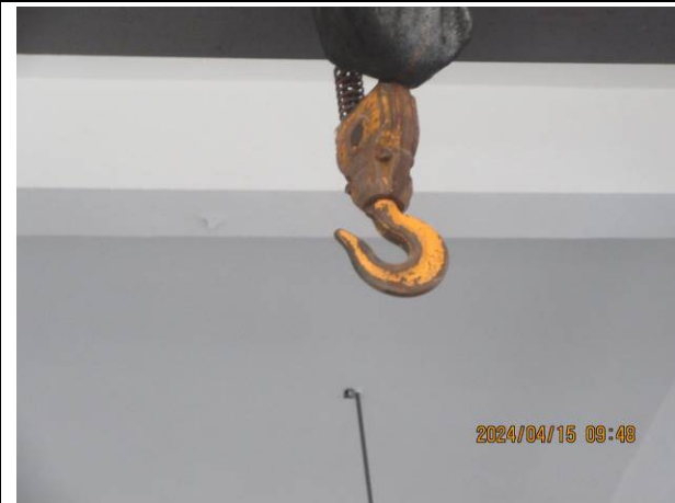
NC7.17 One crane's hook missed safety buckle
